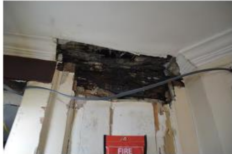
01 Opening up works. Rotting timbers in Room 2 ground floor of Woodcote Cottage caused by water ingress at second floor roof level.
