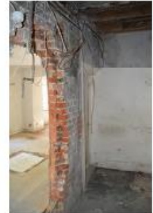
04 Unauthorised works. View inside Room 14 of the original stable block opening, widened.
